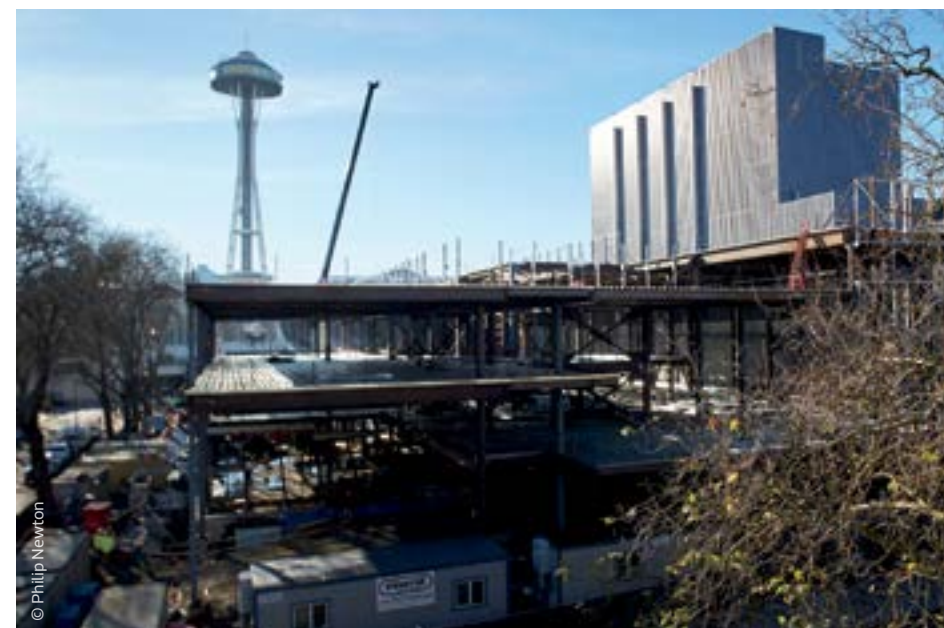
Ideally located, the Opera Center joins fellow arts organizations and cultural attractions on the Seattle Center campus.
