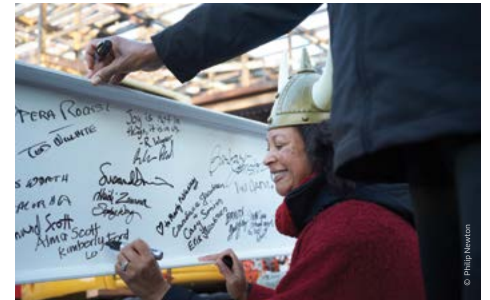
Near the end of 2017 friends of Seattle Opera celebrated another construction milestone by adding their signature to one of the last beams to top the 105,000 sq. ft. arts facility.
